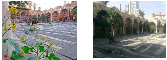
Figure 1 – corrugation in the soil surface under the slabs in SoulimanTikie
