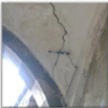
Figure 2 – Cracks in the cupolas of Souliman Tikie
