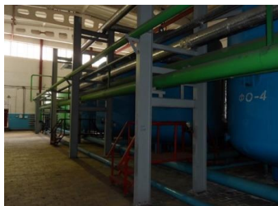
Figure 1 – Chemical water treatment workshop of TPP-1 in Semey
